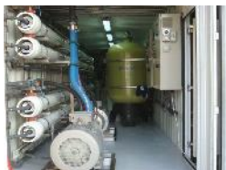
Containerized Seawater Reverse Osmosis Desalination System
