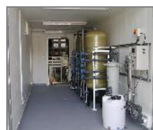
Containerized Filtration/ Disinfection System
